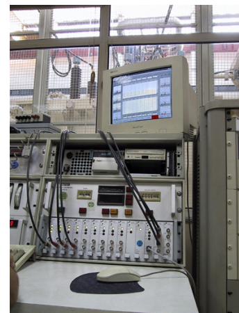
ICMsys8 installed in a control room
